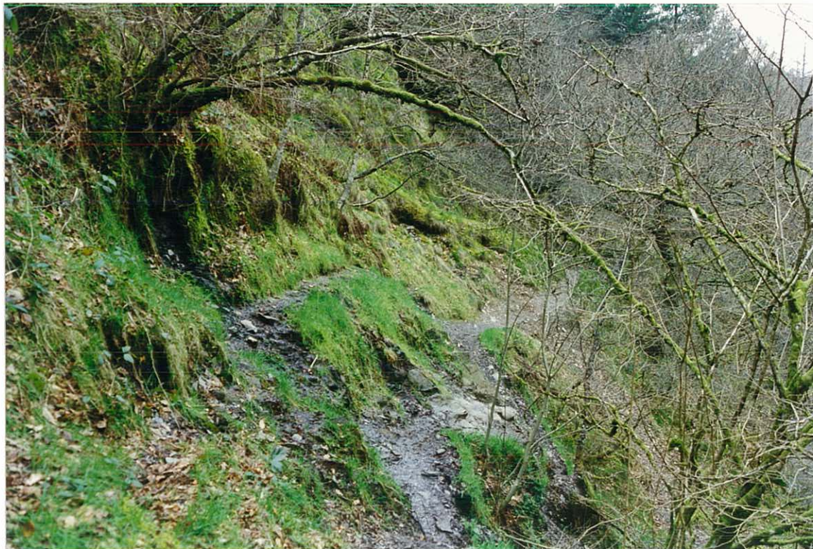
Photos. 1 & 2. North of the old mine level. Prior to the remedial work. The overgrown terrace of Gentleman's Walk can be seen with the worn modern path below.
