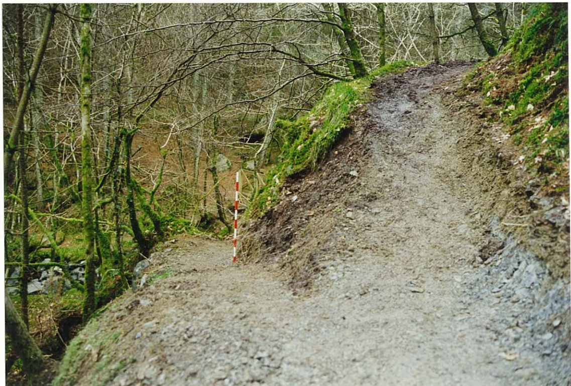
Photos. 9 & 10. Remedial work on the path at the junction of the Gentleman's Walk and the path down to the footbridge over Nant Cau
