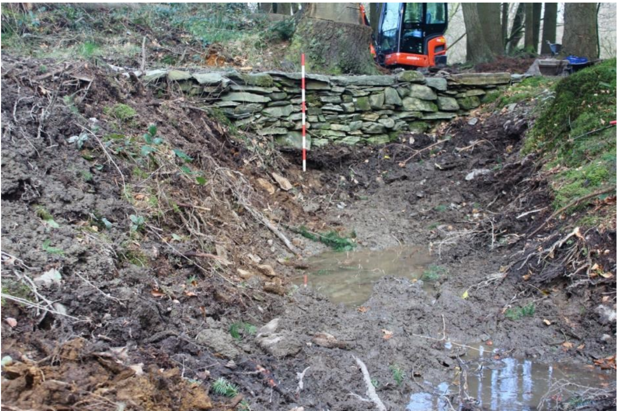
Photo 2: The leat and the modern-built pathway over it, with a 1m scale, after excavation
