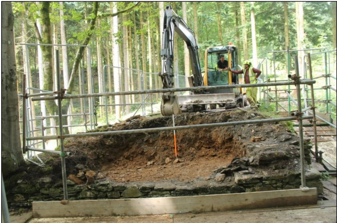
Photo 20: The section of the abutment infill and the reduced walls at the end of the excavations of the north-western abutment (DAT Photo 110511_0038).
