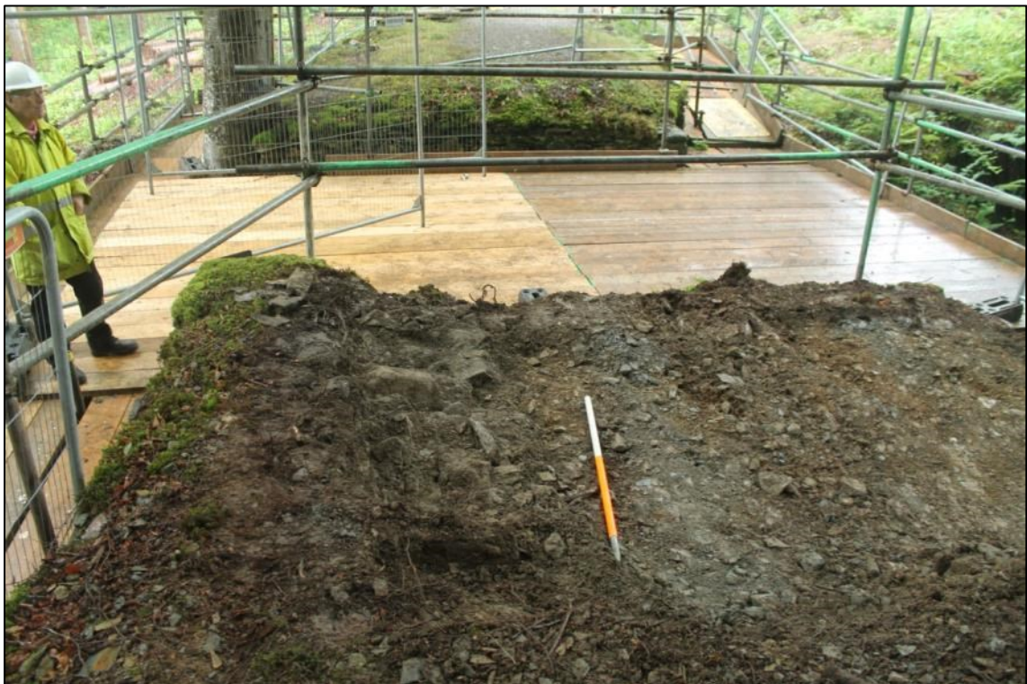
Photo 4: The internal wall line of the southern wall of the south-eastern abutment was revealed after removing the compacted grey deposit (102). A remnant of this is still visible to the right of the ranging pole (DAT Photo 110511_0009).
