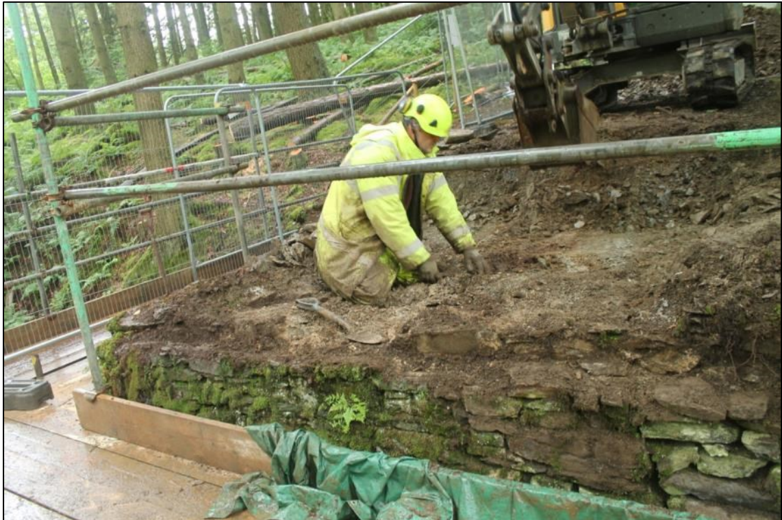
Photo 6: The insert for the bearing beam on the western face of the south-eastern abutment. The height of this wall was reduced by hand (DAT Photo 110511_0014).
