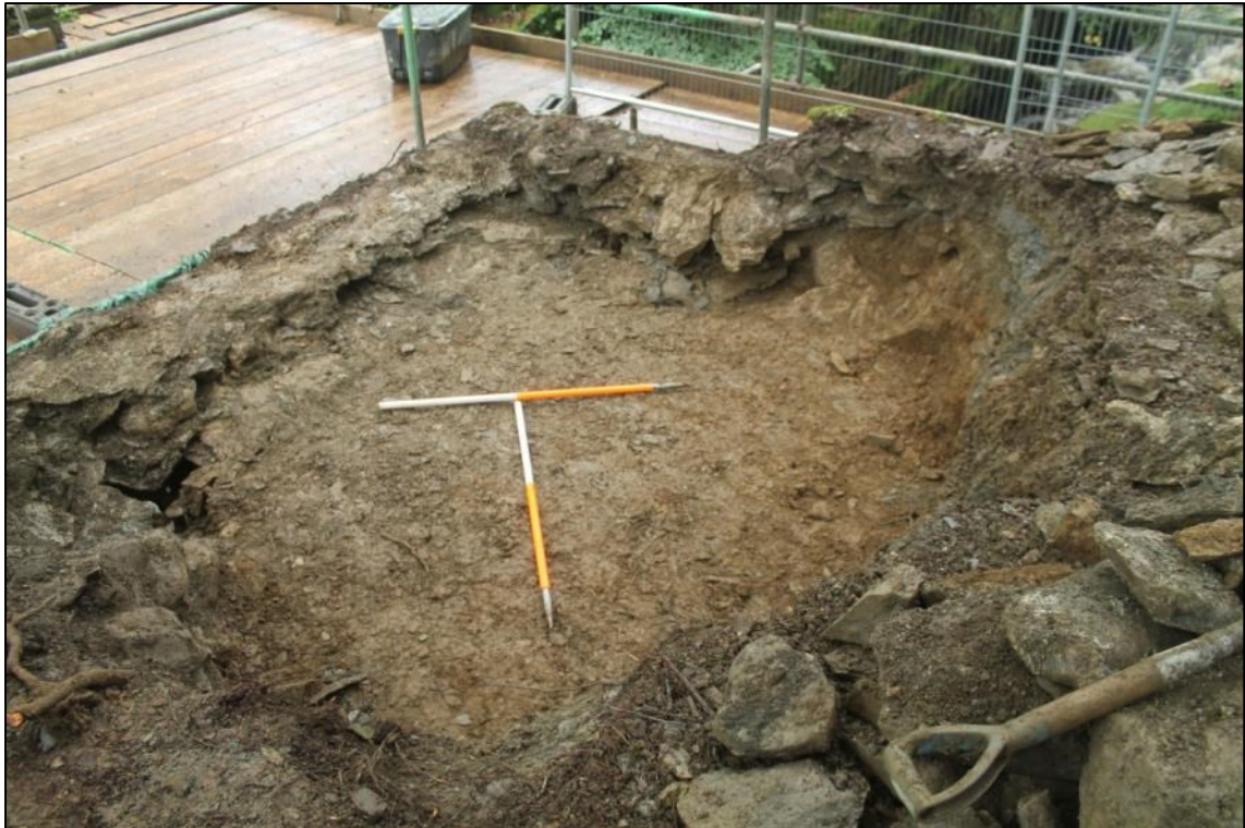
Photo 10: An overview of the final extent of the excavations in the south-eastern abutment showing the partially dismantled western and northern walls of the abutment (DAT Photo 110511_0030)
