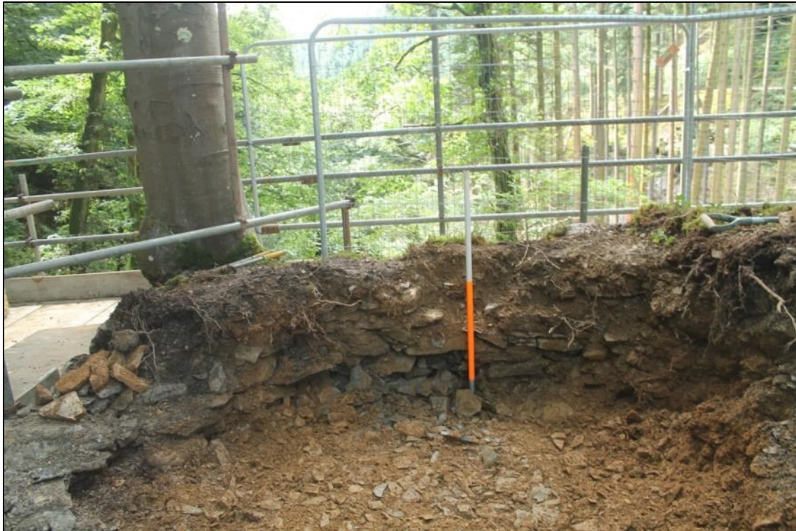
Photo 18: The root damaged southern wall of the north-western abutment (DAT Photo 110511_0041)
