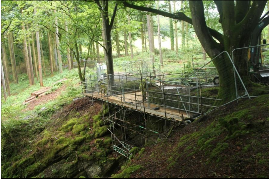
Photo 1: The scaffolding platform erected around Pont Newydd abutments. View facing north (DAT Photo 110511_0021)
