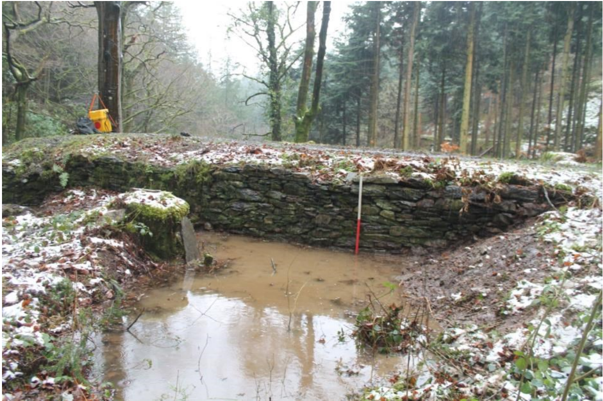
Photo 3: North-eastern facade of the northern abutment exposed during the evaluation. 1m scale
