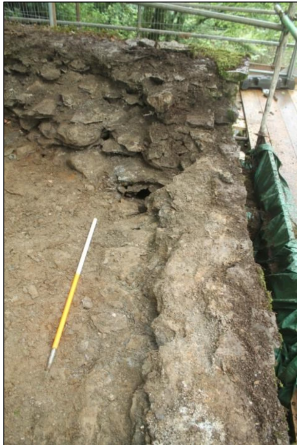
Photo 9: The partially dismantled western wall and southern return wall of the south-eastern abutment (DAT Photo 110511_0028)
