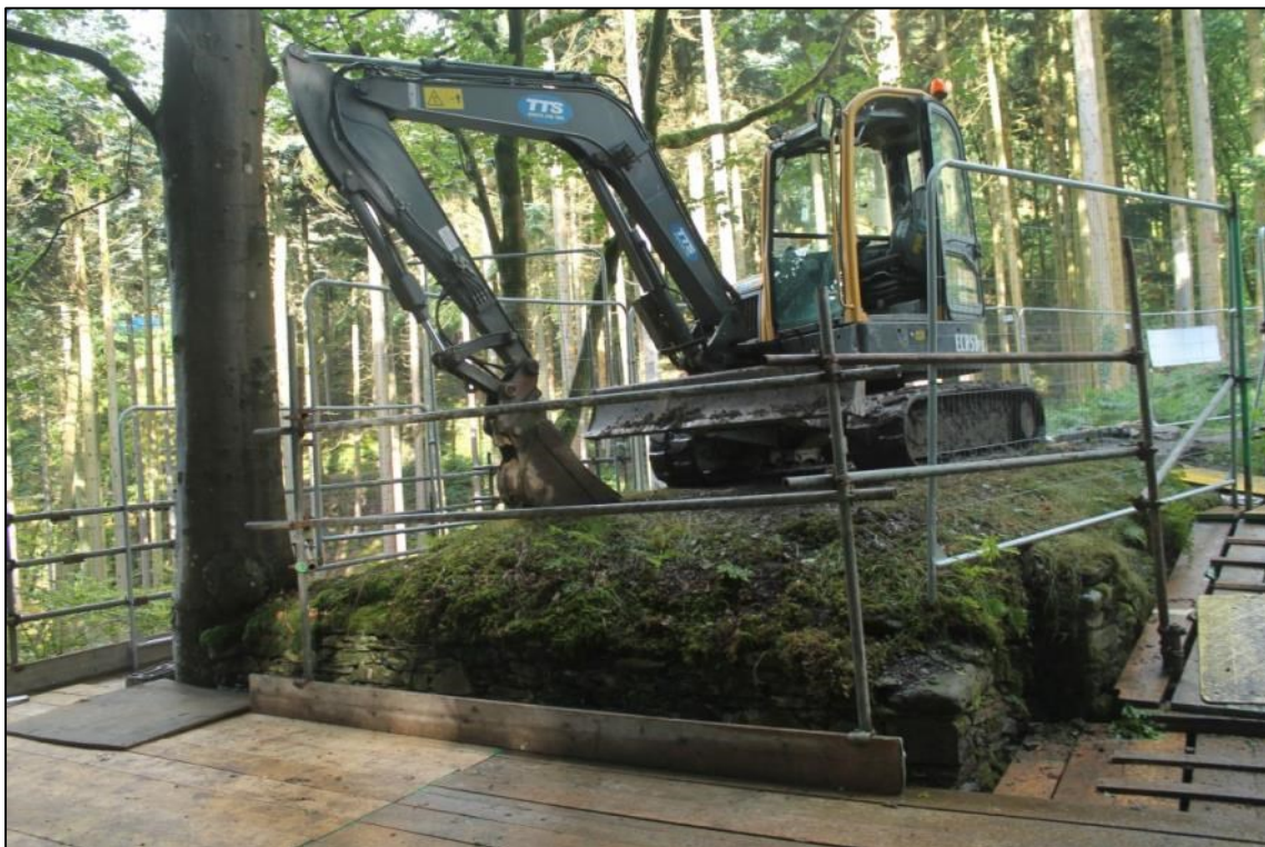
Photo 12: The north-western abutment prior to the start of works. Note the dogleg inset along the northern wall of the abutment (DAT Photo 110511_0031).
