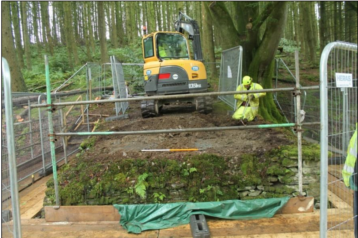
Photo 3: Removal of the surface deposits revealed the former carriage-ride surface. This had been truncated by a test pit in the centre of the abutment (DAT Photo 110511_0006)
