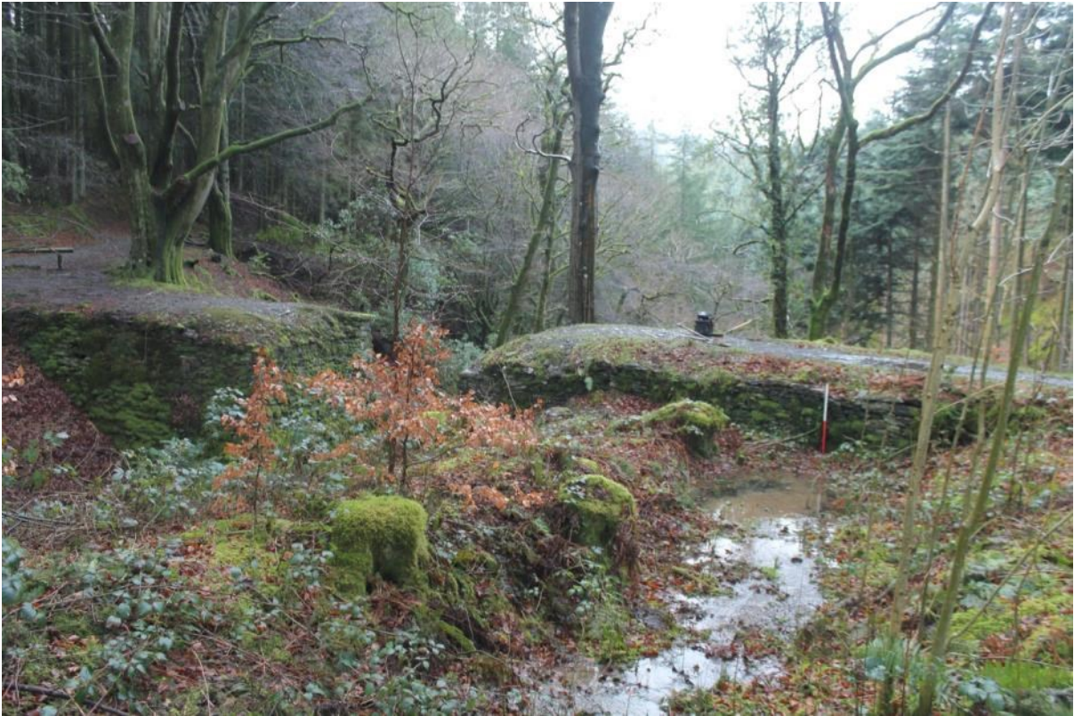
Photo 1: View east showing both bridge abutments of Pont Newydd following tree clearance
