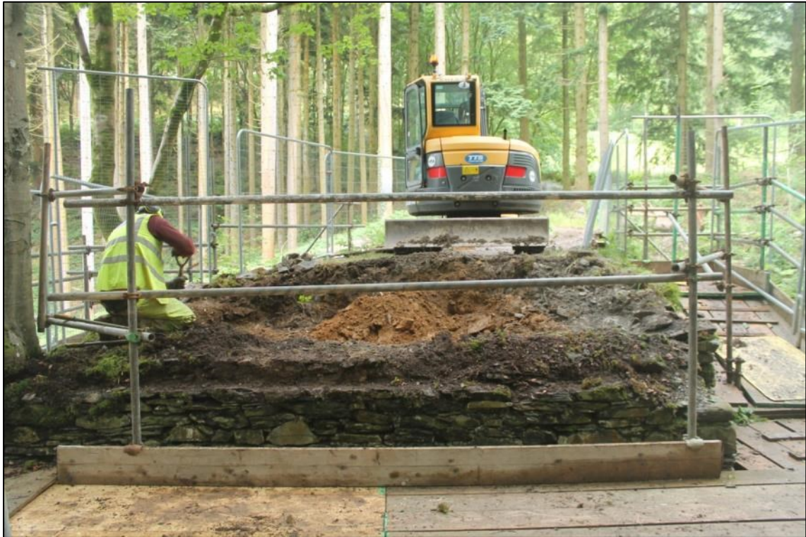
Photo 15: The bearing beam inset revealed on the eastern wall of the north-western abutment (DAT Photo 110511_0035).
