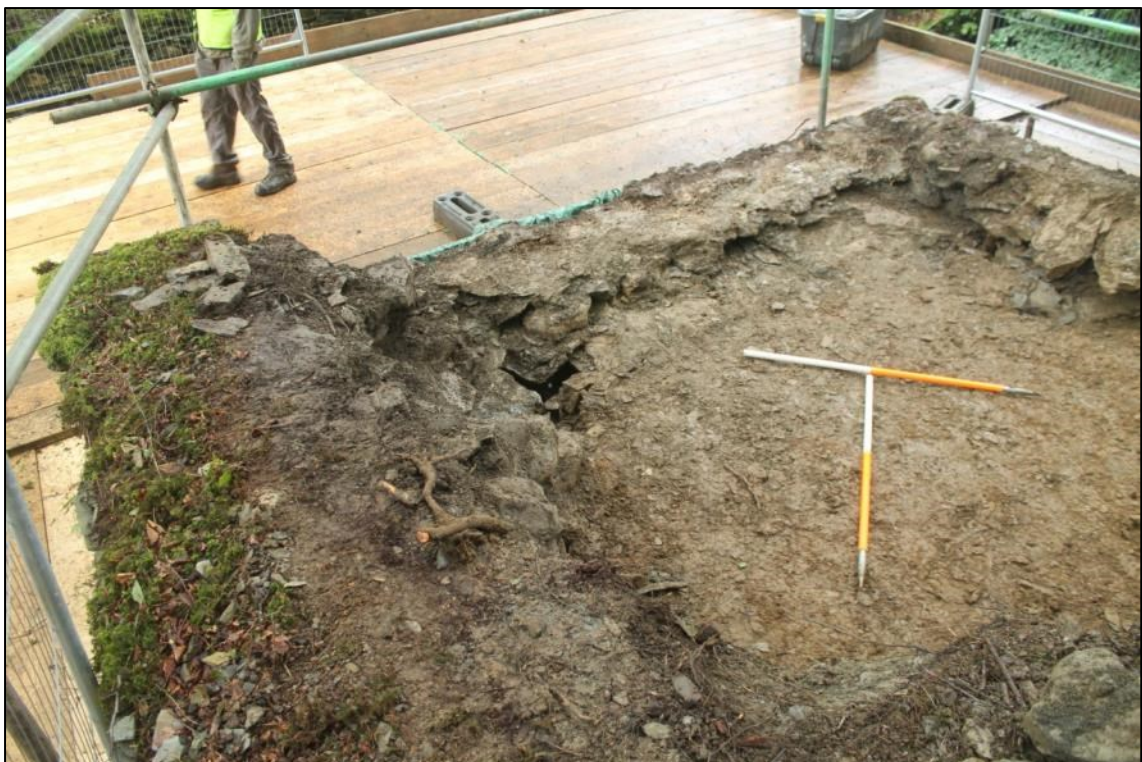
Photo 7: Overview of the final extent of the excavation in the south-eastern abutment. The extent of the southern wall is shown in the left side of the photograph (DAT 110511_0029)
