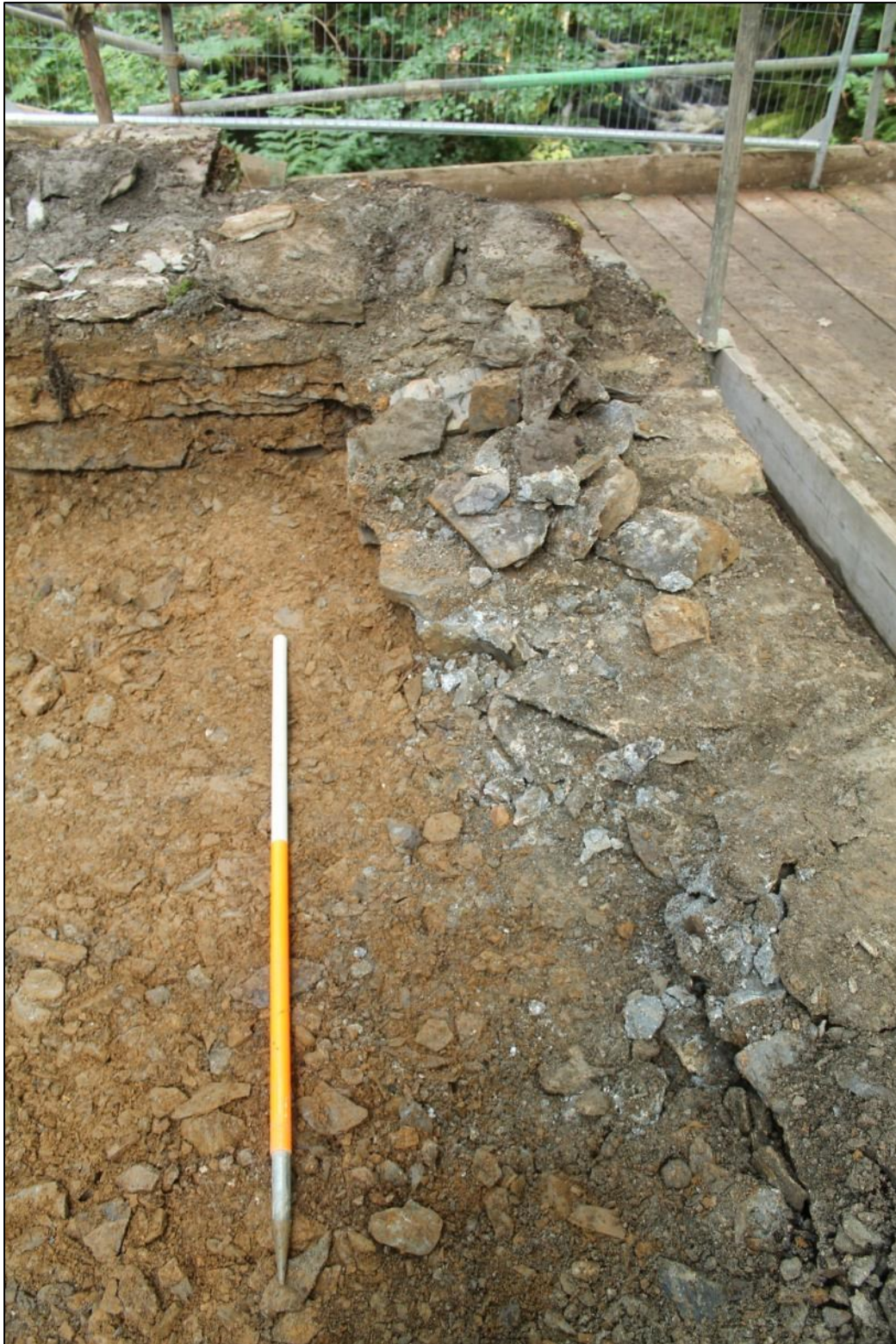
Photo 17: The corner of the northern and western walls of the north-western abutment (DAT Photo 1105511_0043).
