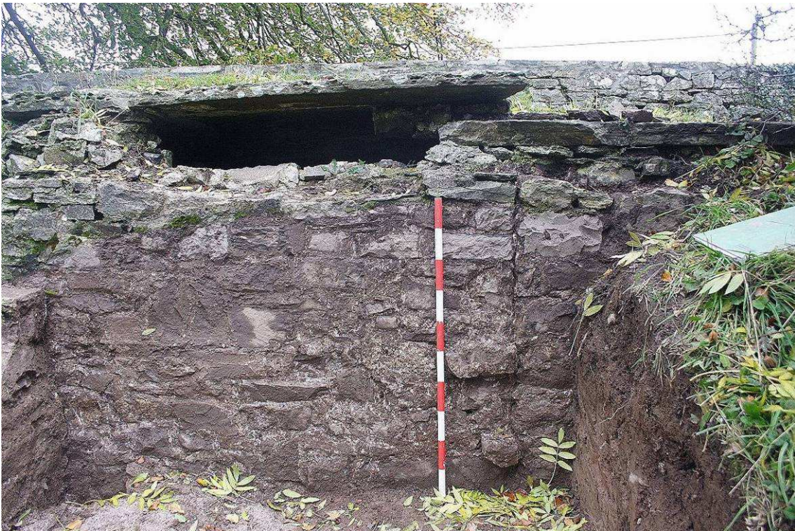
Photo 13: WNW facing shot of the eastern wall of Rooms 1 and 2, showing the construction break on the right. 1 x 1m scale
