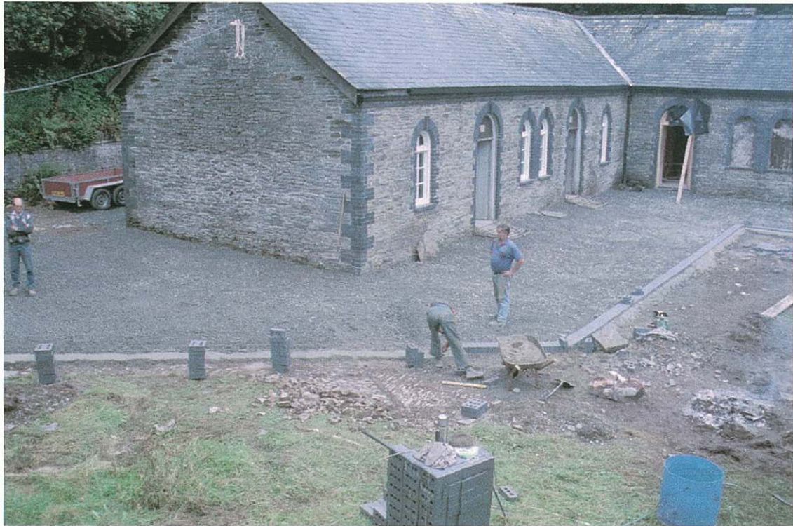
Photograph 6. View of stable courtyard looking north during laying of stone apron. Pitched cobbling (O) in foreground.
