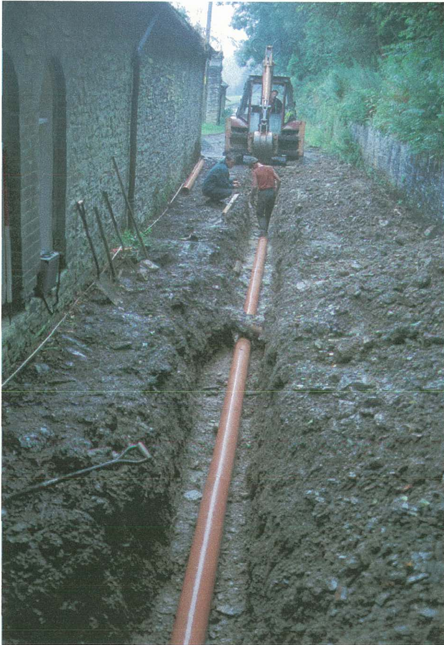
Photograph 2. Working shot during excavation of sewerage pipe trench on north-west side of stable block.
