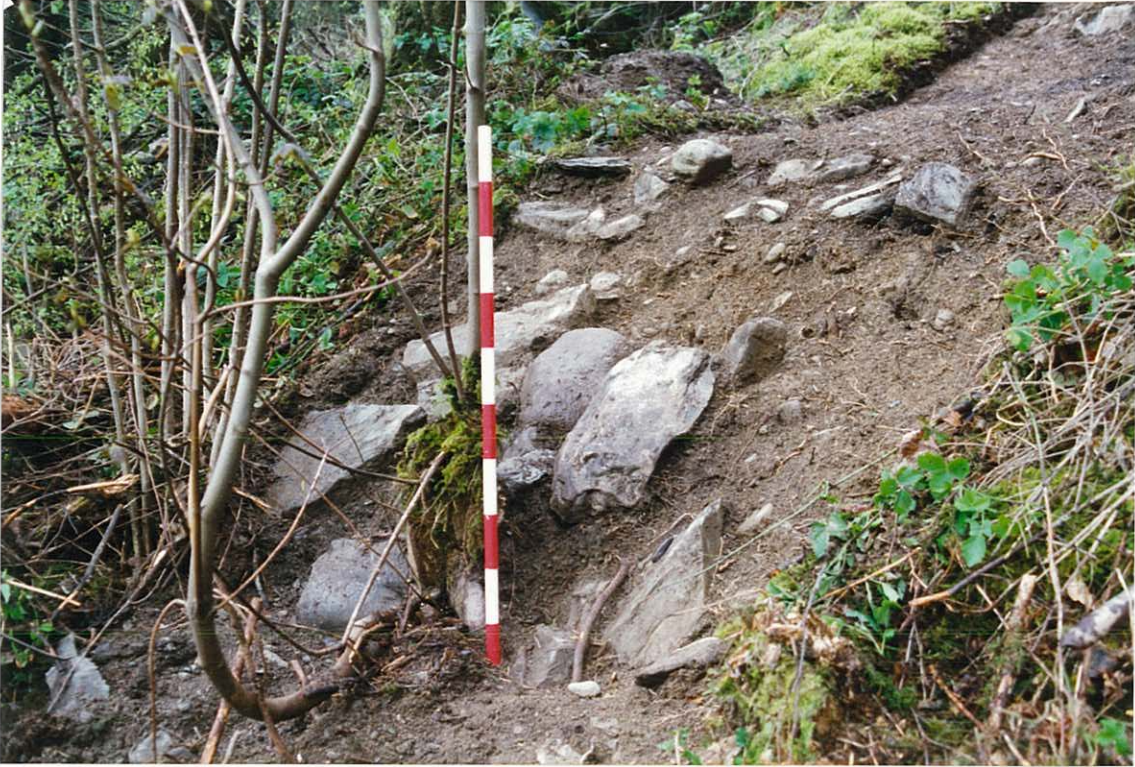
13. Trench 3 showing collapsed revetment.
